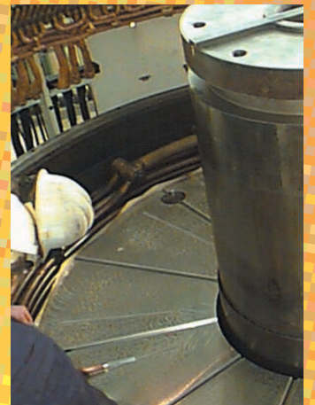
Large installations are a Kingsbury specialty.
