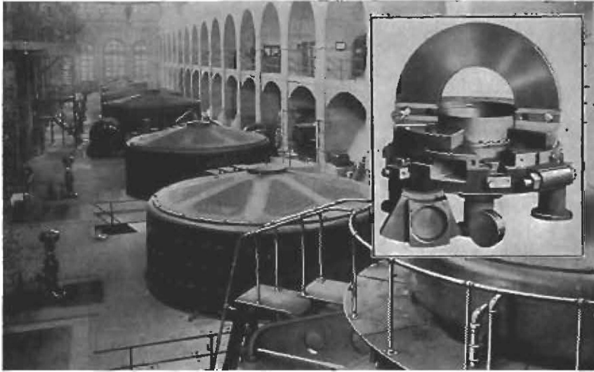
Holtwood Station of the Pennsylvania Water & Power Company. Kingsbury Thrust Bearings are 48 and 56 inches diameter. They are of the adjustable (not equalizing) type. One of them is shown in the inset, with one shoe removed and one-half of split runner turned up on edge. Installed 1912 to 1924.
