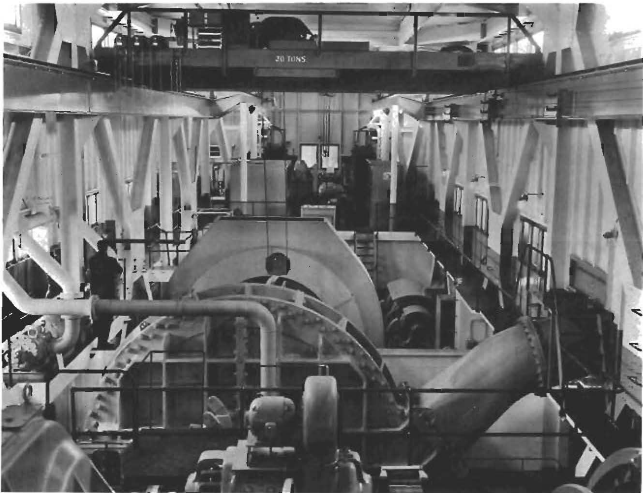
View of the Engine Room of the dredge "Hydro-Quebec" showing the machinery of one of the world's largest Pipe Line Dredges, an important production unit in the dredging of the Beauharnois Canal, part of the St. Lawrence Waterway System.
